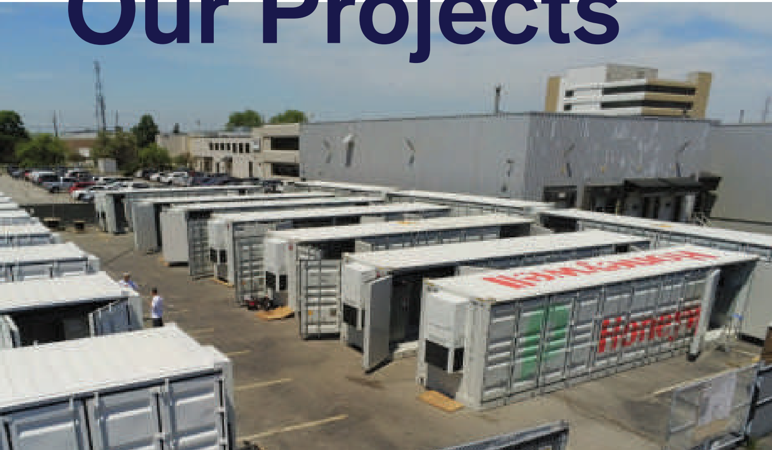
Ontario • Over 150MWh of Global Adjustment Integration and EPC Services | Partner: Honeywell
