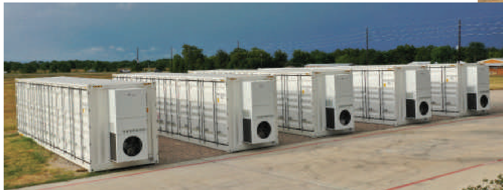
New York • 12.5MWh NYSEDA BESS | Partner: Key Capture Energy (KCE)
