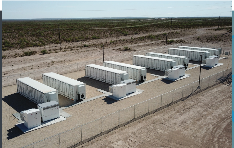
Pictured: Texas Manufacturing Facility Engineering, Design, Integration for 100 MW/ 100MWh installation. Ontario: Over 100 MWh of assets under contract for O&M services with a global leader in infrastructure services.
